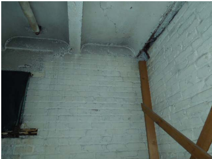
Photo #11: In the basement storage room directly off the boiler room, there is a crack in the ceiling pan aligns with a crack in the brick wall. We recommend these cracks be investigated and corrective action taken as necessary.
