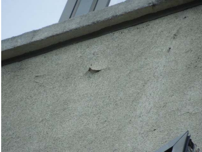
Photo #13: Stucco deterioration on south wall of building. This should be corrected to prevent further deterioration.
