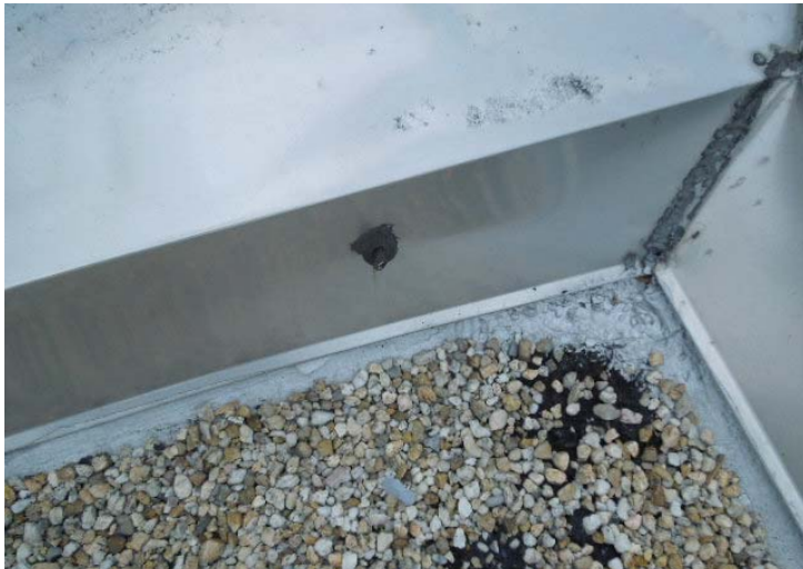
Photo #5: Nails backing out of cap flashings should be secured and caulked to maintain the seal and prevent further damage.
