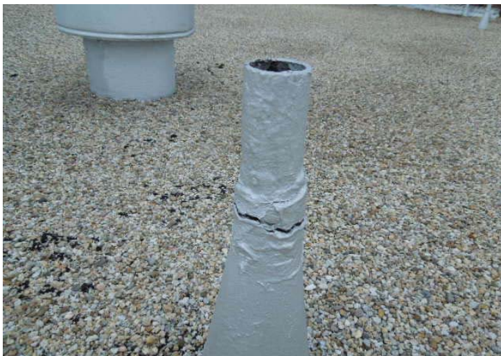
Photo #6: Vent flashing sealant has deteriorated. This can allow water to follow the outside of the piping into the building. We recommend these flashings be sealed.
