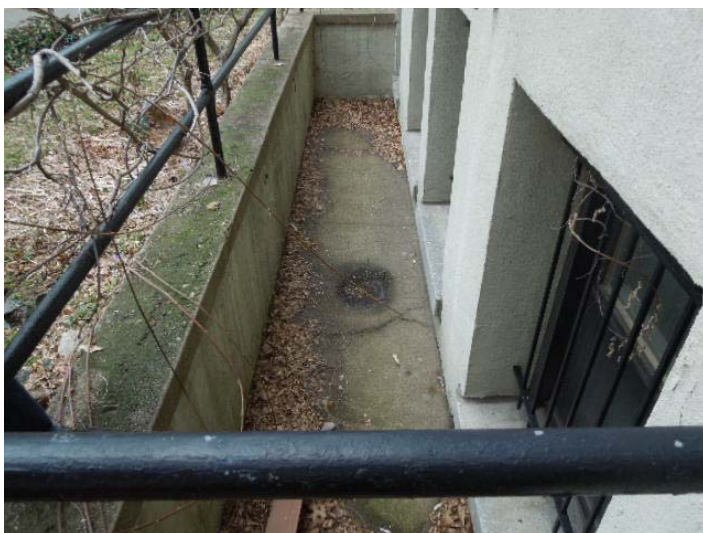
Photo #12: We recommend that the window well be cleared of leaves and debris, and that the drain be cleared so that water will not fill the well and potentially leak into the building through the windows.
