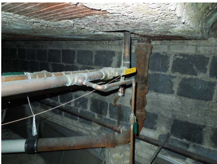
Photo #9: Typical ball type isolation valve on the domestic water riser in the crawl space. This is the recommended type of valve.
