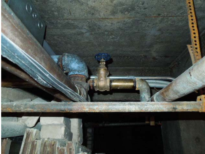
Photo #10: Typical gate type isolation valve on the domestic water riser. These valves tend not to seal for as long.
