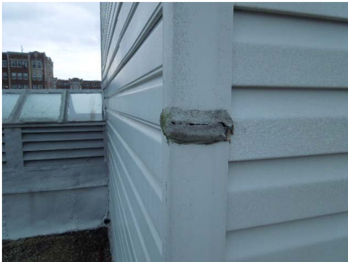
Photo #8: Caulk is failing on vinyl siding of penthouse. We recommend this caulk be replaced.
