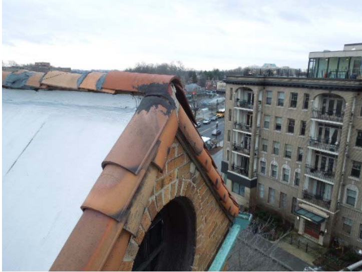
Photo #4: Cap tile is cracked. Tile sealant has deteriorated on west side gable cap.
