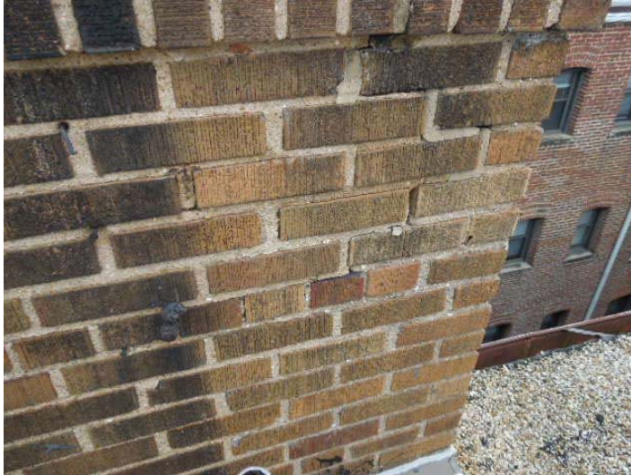
Photo #7: Point work failing and cracking on chimney. This could be latent earthquake defects. We recommend this be pointed and sealed to prevent further deterioration.
